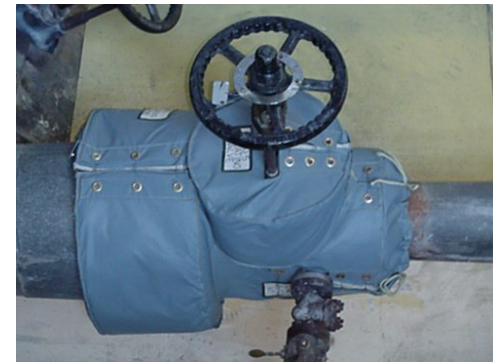
Steam valve with cover installed
